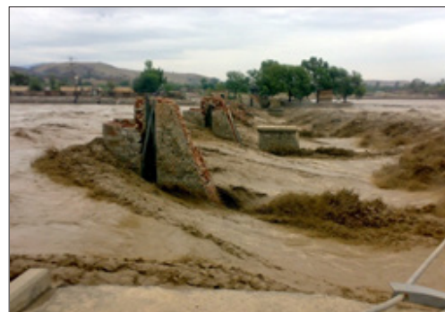
Figure 24: Munda Headworks Structure destroyed after flood 2010 [50]
