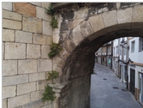
Figure 10: Flight of a quadcopter drone during the inspection of a singular point of the Roman Wall of Lugo; specifically in the Porta de San Pedro ou Toledana and images captured by the drone, where the deterioration of the stone material can be observed (photographs by the author).
