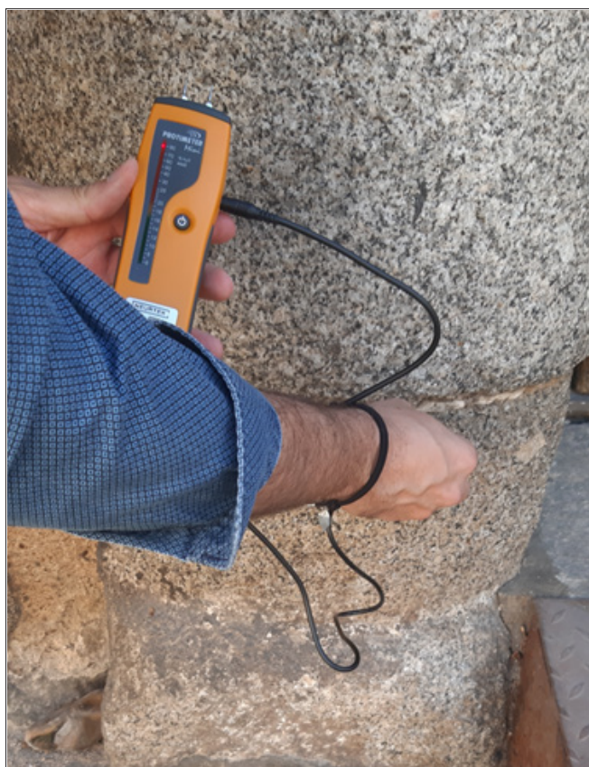
Figure 11: Humidity measurement using a protimeter in the columns of the access gate to the Palace of King Don Pedro
