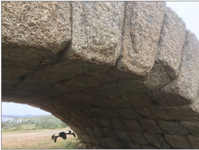
Figure 3: Quadcopter drone circulating inside the first vault of the Roman Bridge of Alconetar (Spain), for inspection of its intrados (photo by the author).
