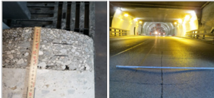
Figure 1: (Left) Pavement stratigraphy. (Right) Rutting along the highway lane.
