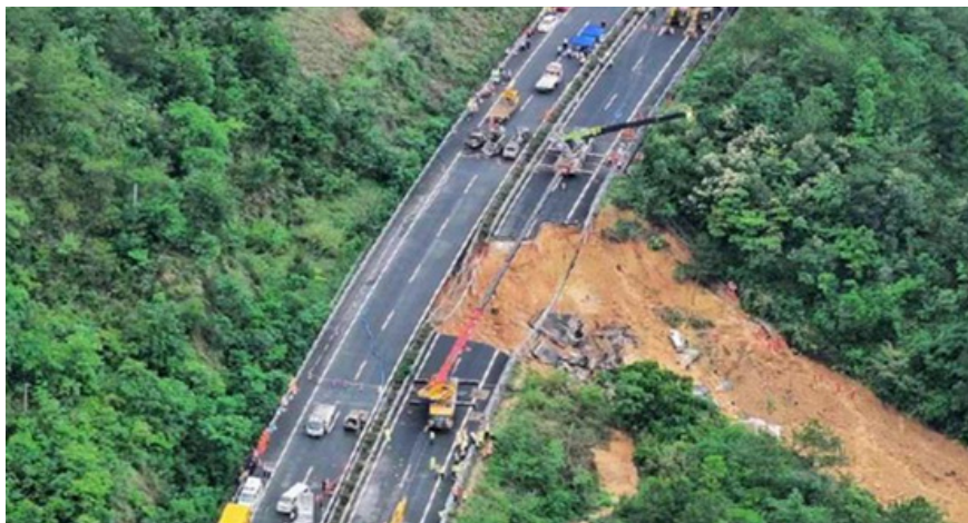
Figure 4: At around 2 o'clock on May 1, 2024, the Chayang section of Meida Expressway in Meizhou City, Guangdong, China, collapsed. By 14:00 on 2 May, 23 vehicles had been found down and 48 people had died.
